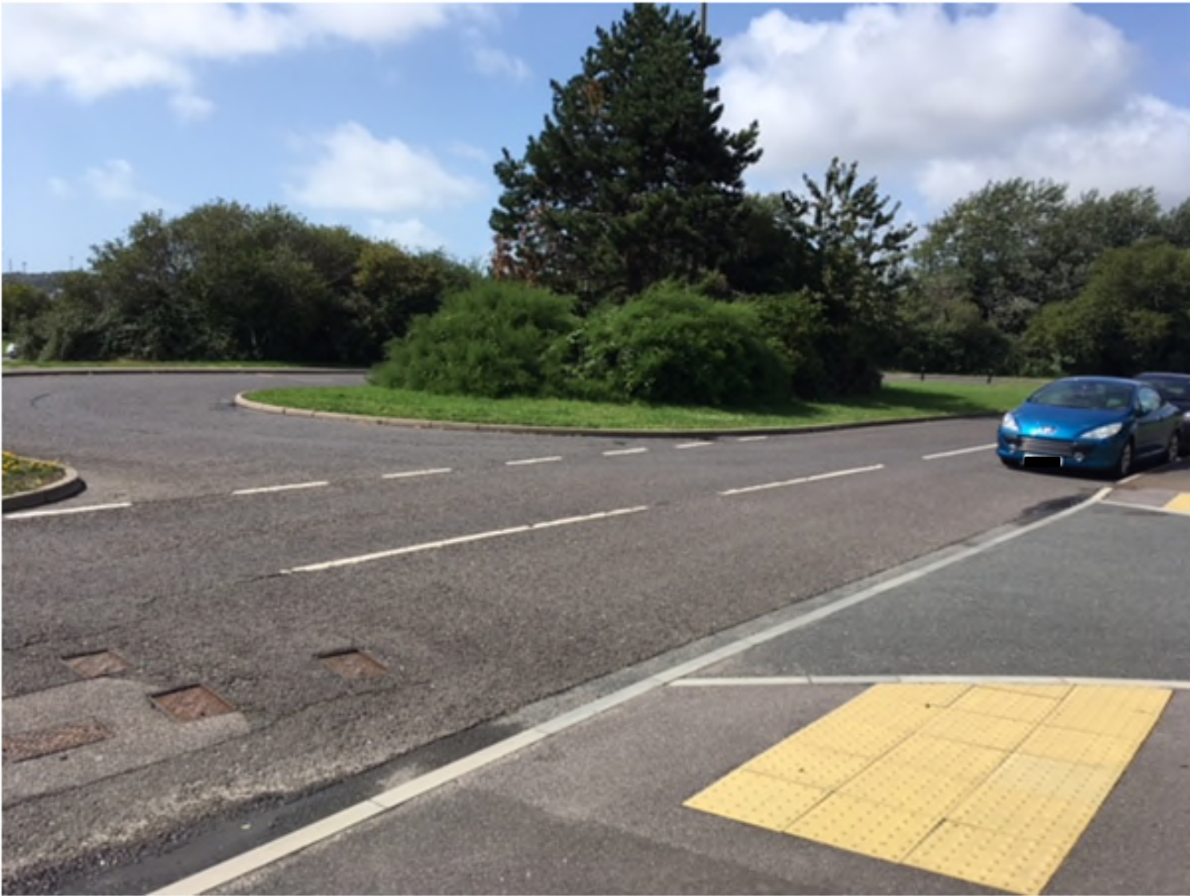
View 2 – Looking south-westwards along Mount Road from the entrance to Tide Mills View
